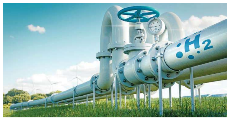
The future use of green hydrogen in Trinidad to produce ammonia and methanol is inevitable
